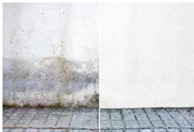
Cemento armato deteriorato Deteriorated reinforced concrete
